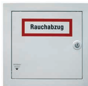
SHEV motor control central including accumulators for backup power supply
